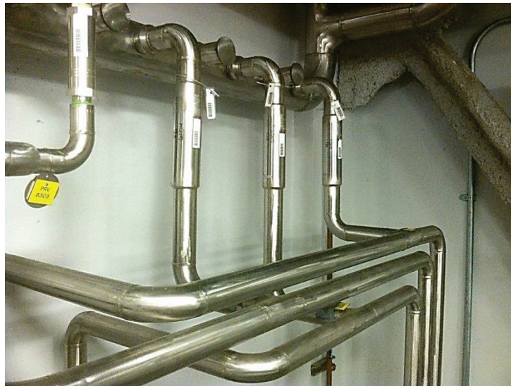
Fig. 4.25. FTS welded pressure relief rupture discs and manifold.
