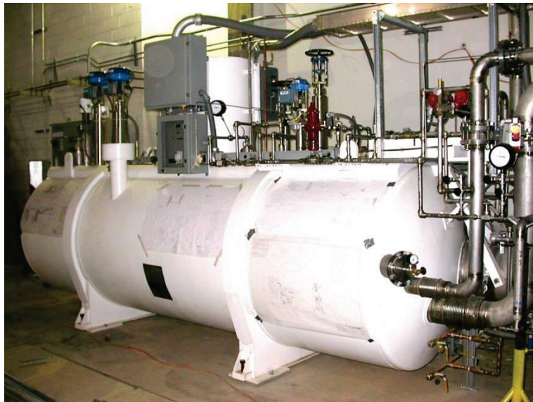
Fig. 4.26. FTS helium refrigerator.
