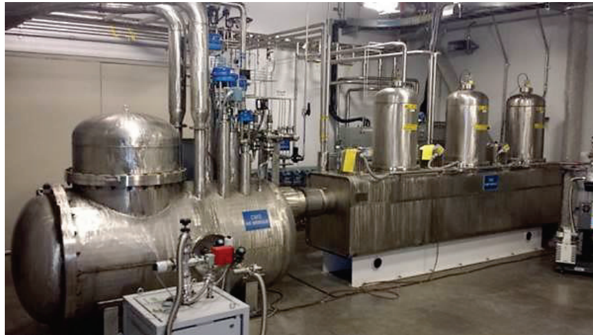
Fig. 4.23. FTS cryogenic heat exchanger and pump modules.
