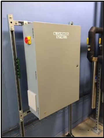
Figure 3: Control panel for slits
