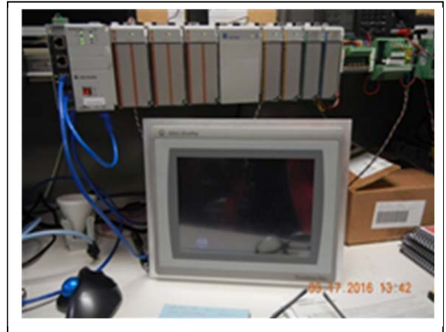
Figure 1 PLC hardware for interlock
