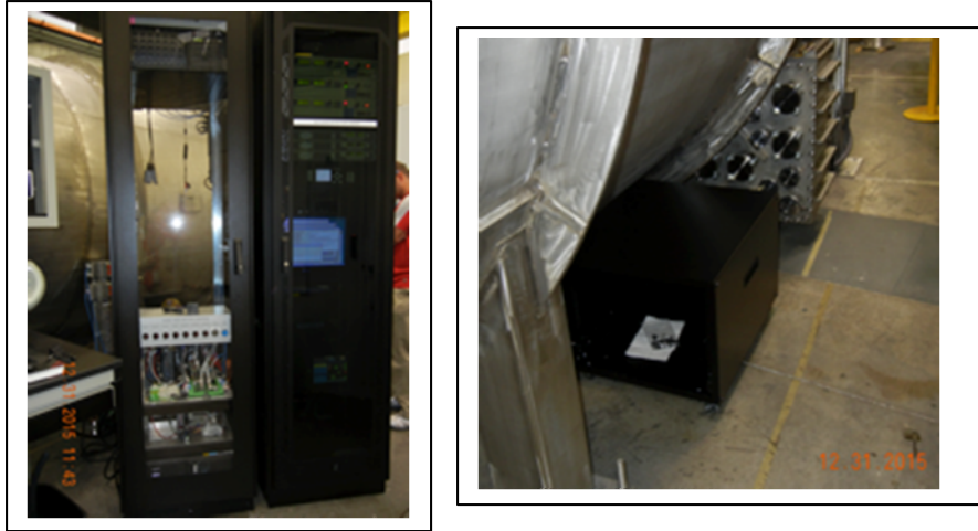
Figure 13: DAS equipment installed
