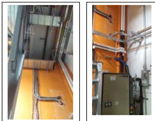
Figure 2: New utility penetrations, cabling, cable tray and vacuum lines outside the ARCS basement
