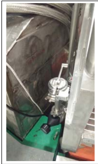
Figure 4: New mechanical vent valve installation with additional access port (below) for vacuum troubleshooting. Located in the sample room, it will pop open when the sample chamber vents, providing a clear indicator that sample chamber has been vented for sample changes.
