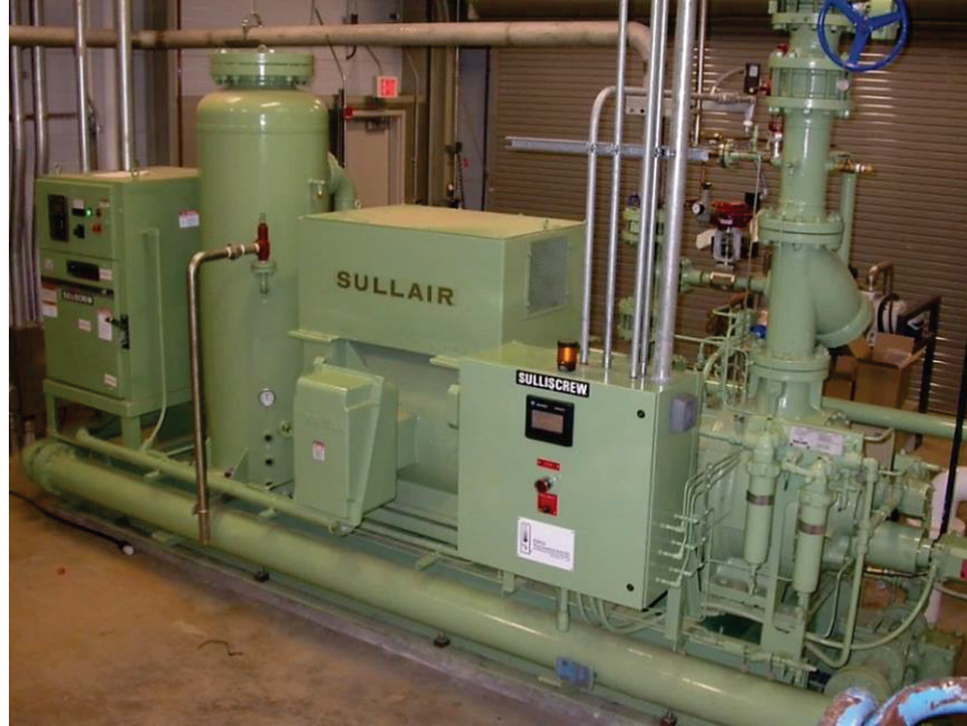
Figure 4.104. FTS helium compressor.
