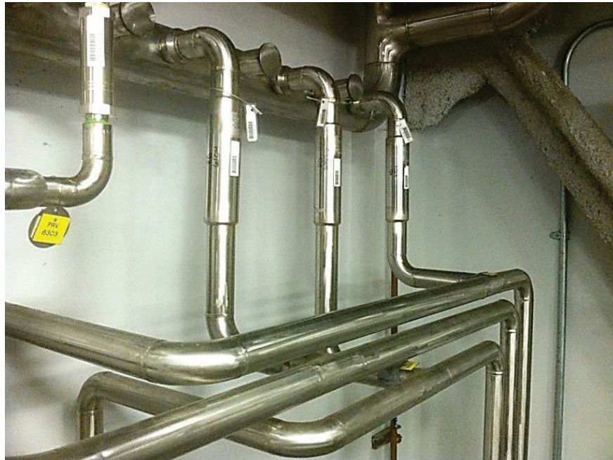
Figure 4.102. FTS welded pressure relief rupture discs and manifold.
