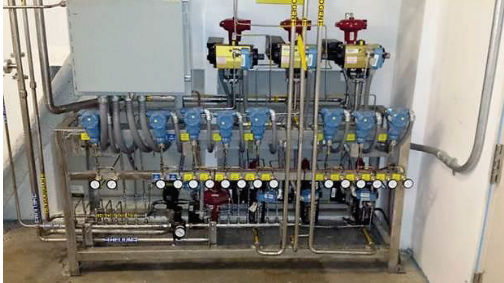
Figure 4.101. FTS Hydrogen gas management system.
