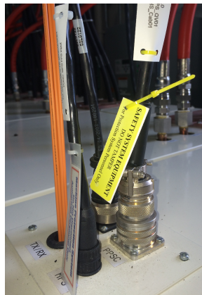
Figure 2 Typical PPS connection at a non critical device magnet power supply. This connection will be removed and a jumper connector installed.
