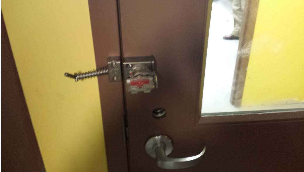
Figure 6. PPS Trap Key Door Lock Mechanism with Jz Key Installed on USANS Instrument Enclosure South Side Entry Door
