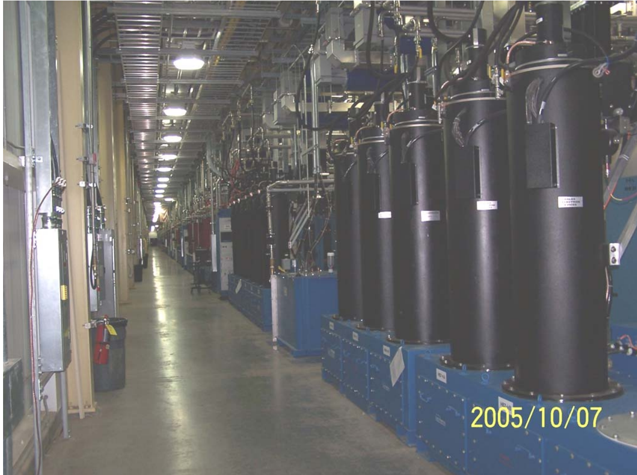
Figure 3.2.1.2-1 Klystron Gallery (from within the superconducting section, looking west)
