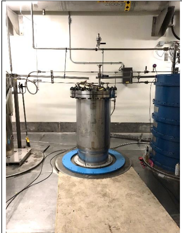
Figure 4: PPU MOTS Delay bed in the Gold Amalgamation Room in early stage of installation.
