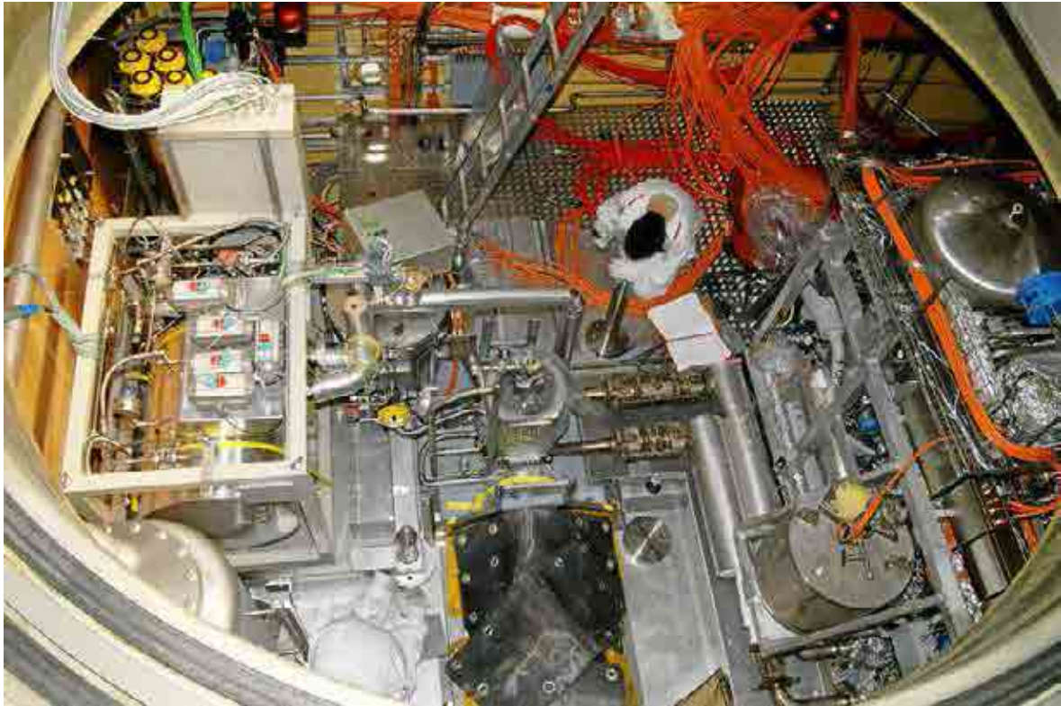
FIG. 4.62. View into the TKE which is on top of the SINQ main shielding block (situation of April 2006). The target head is in the centre, still without the cables connected which are in preparation in the rear, the oil loop of the HRS is at the right, the F&D system at the left, and the CGS in the left rear corner (partly hidden).
