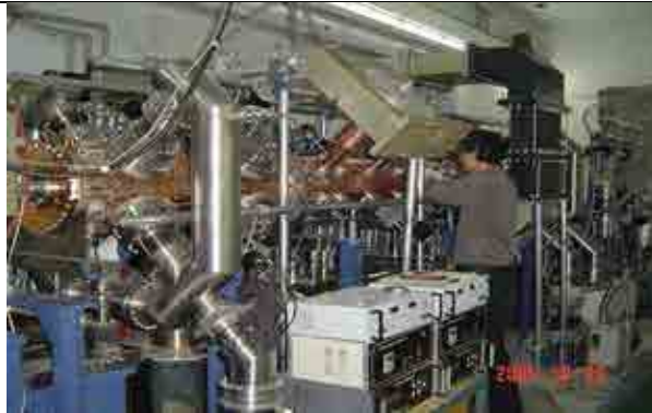
FIG. 4.39. RFQ installed (prior to cooling connection).
