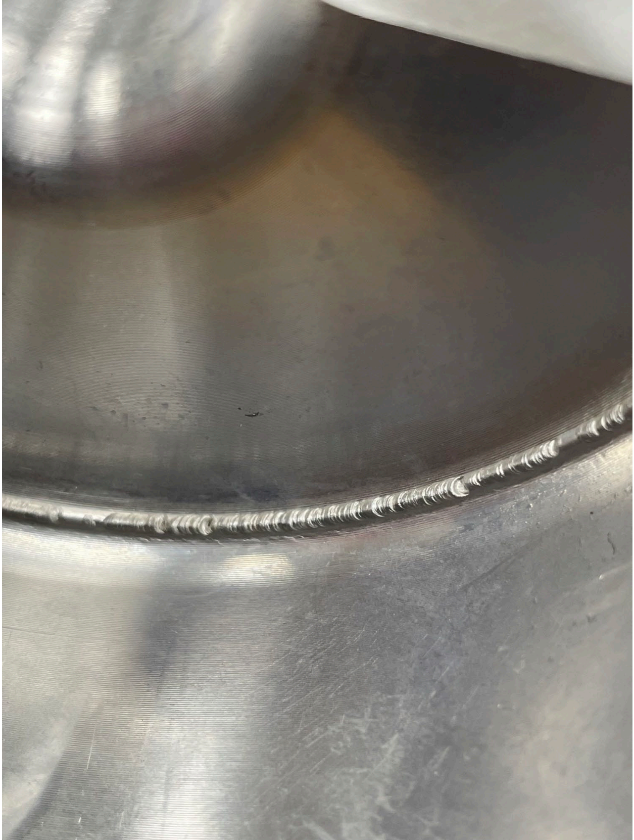
Over penetration of vacuum vessel weld backer resulting in melting of backer.
