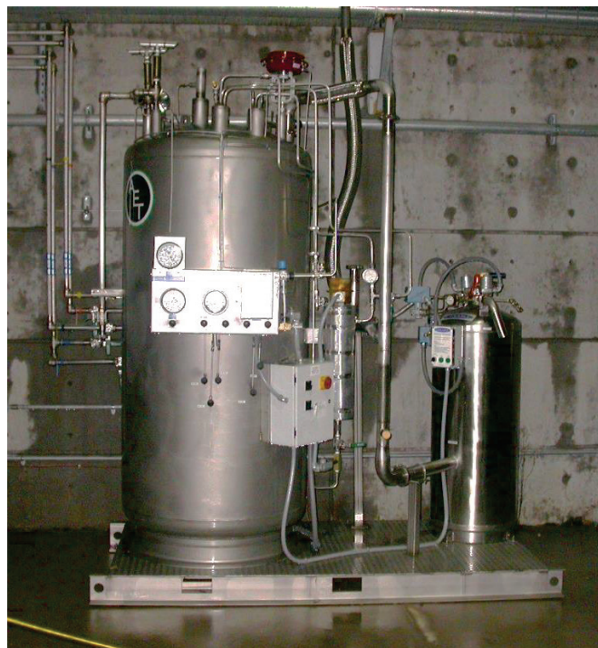
Figure 4.106. FTS helium gas purifier.
