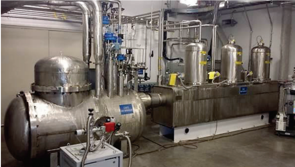
Figure 4.100. FTS cryogenic heat exchanger and pump modules.
