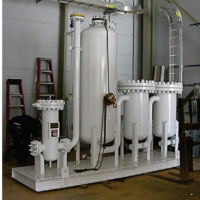
Figure 4.105. FTS oil removal system.
