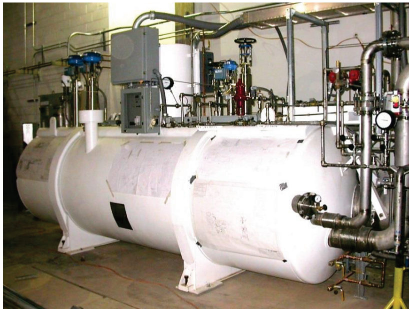
Figure 4.103. FTS Helium refrigerator.
